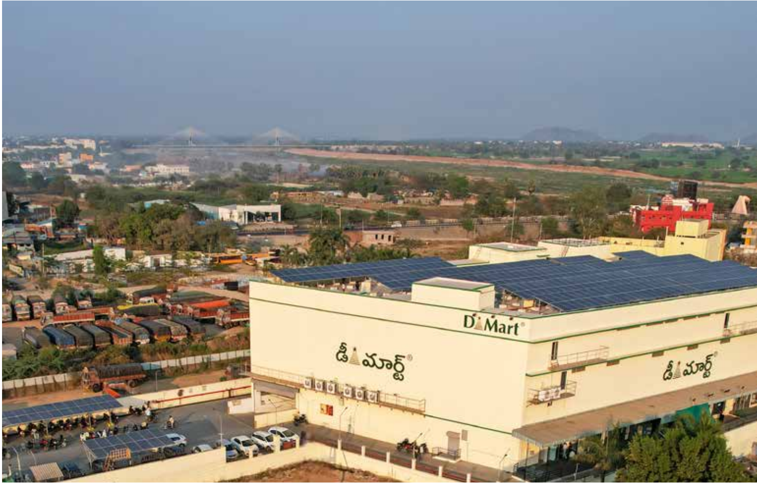
Rooftop Solar Panels and Solar Carports
