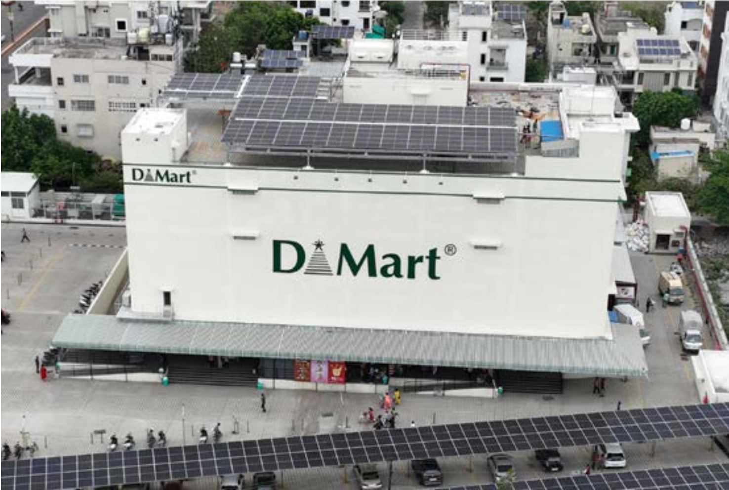
Rooftop Solar Panels and Carports
