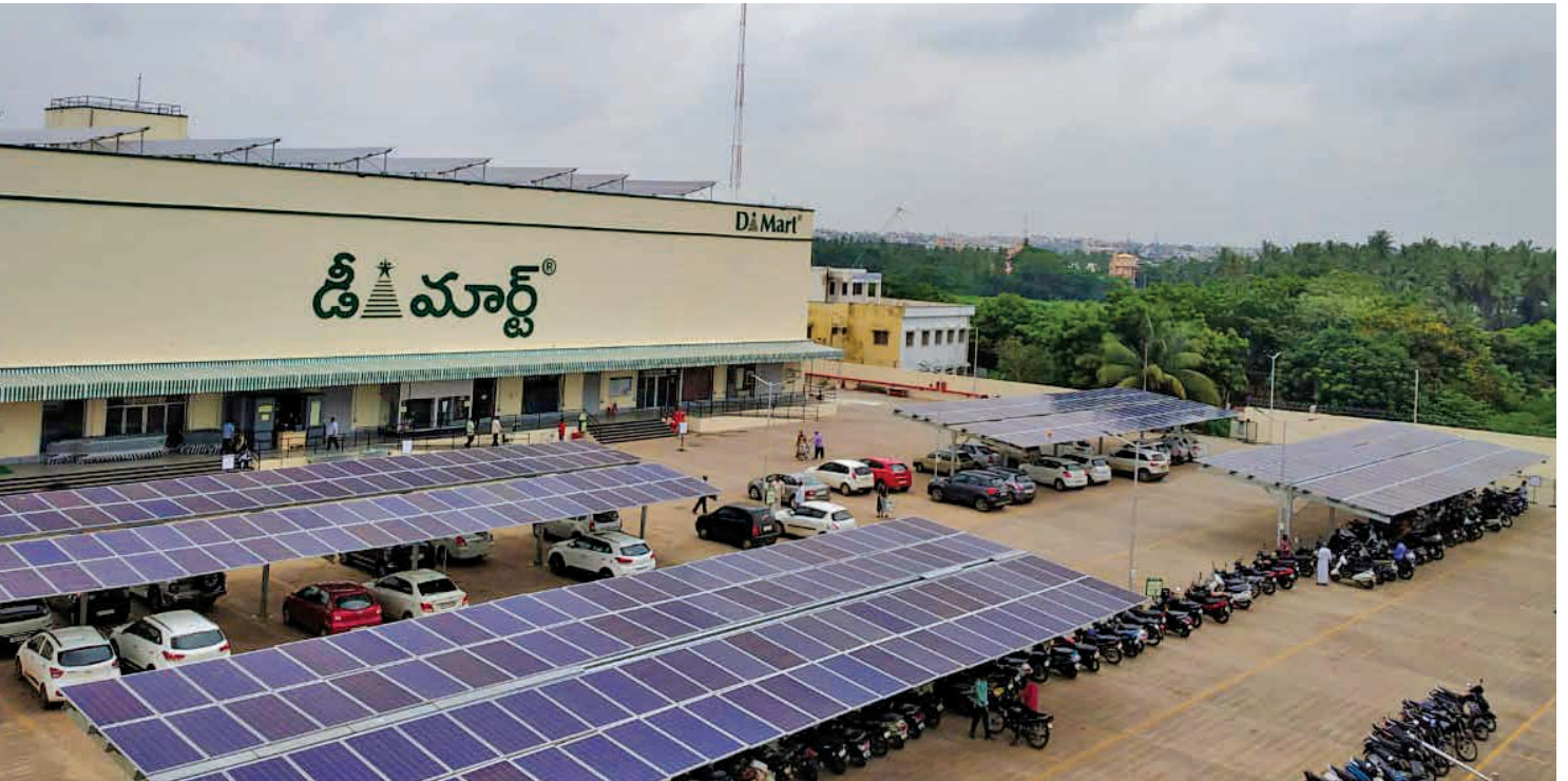
Rooftop and Carport Solar Panels
